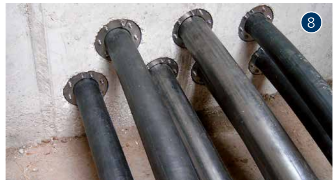
HRD press seals installed
