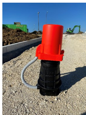
The fully assembled G-Box can be installed in the new-build development as shown. The finished connector can be connected directly to the router via a cable system through light-coloured corrugated pipes.
