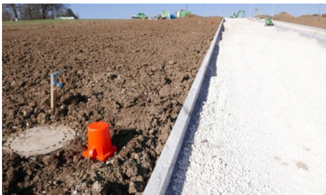
The pylon marker indicates the presence of G-Box, making it clearly visible within the new-build development. The additional lengths of fibre-optic cable can be stored under the pylon markers.
