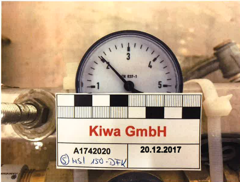
Figure A3. Water tightness test with \geq 2,0 bar water filled test cylinder (manometer at the beginning of testing on 20.12.2017).
