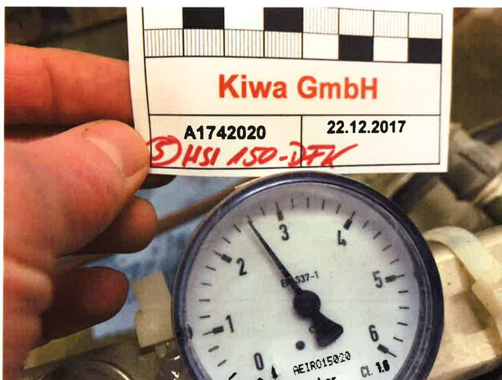
Figure A6. Water tightness test with \geq 2,5 bar water filled test cylinder (manometer > 24 hours on 22.12.2017).
