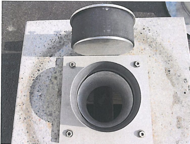
Figure 4: Flange plate with removed HRD 150-2F-0
